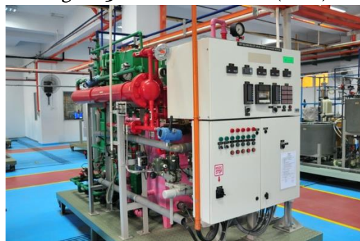
Figure 4. Bolier Drum-Temperature pilot plant with HART Fieldbus system (USM)
