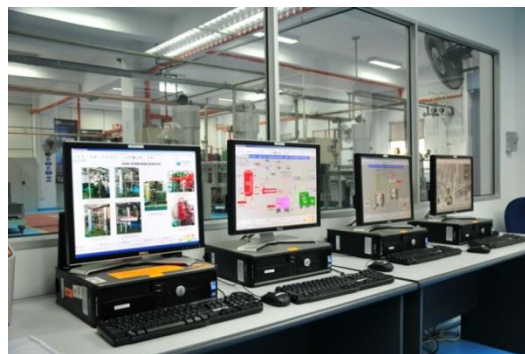
Figure 3. DCS control room (USM)
